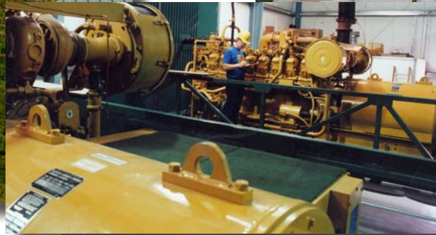
EPUD Short Mountain Methane Power Plant ↓
