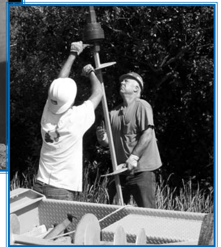
Lineman Brad Trommlitz and Line Foreman Bill Vezina put together 80 feet of anchoring in 50 pound sections to hold a steel transmission pole in place in any type of weather.
