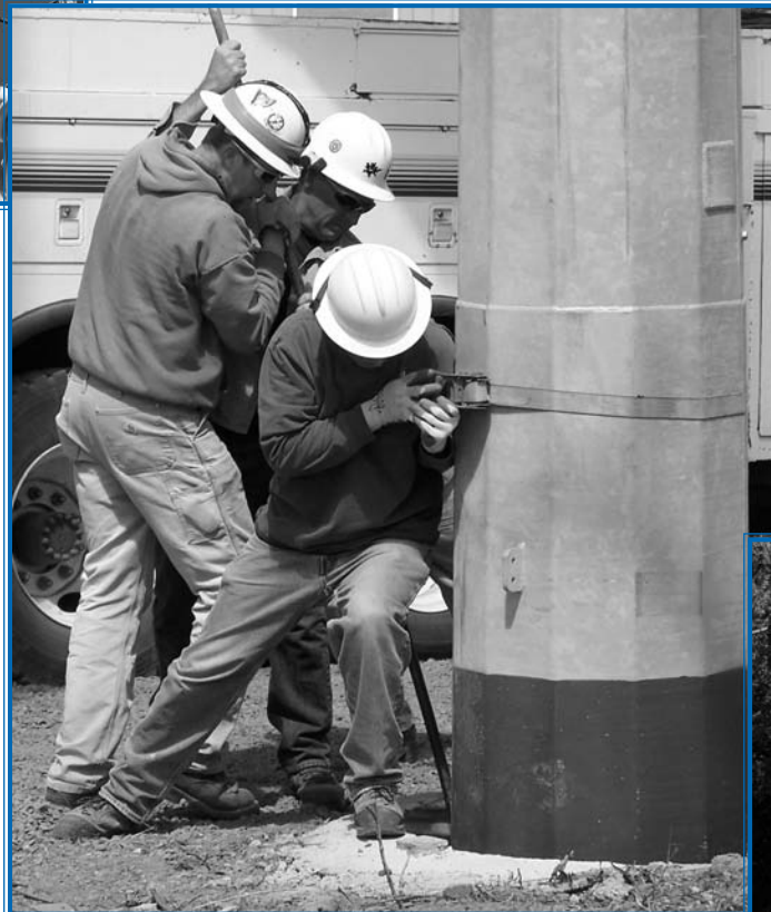
(above, front to back) Linemen Leo Newman, James Barber, and Bob Jolley muscle the base of this three and a half ton steel transmission pole into place. It must be set exactly at the correct vertical.
