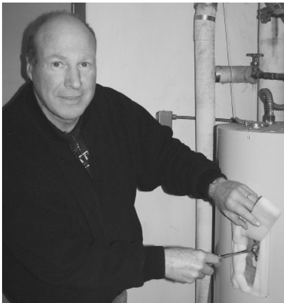
While checking the thermostat in a water heater takes a few steps, Frank in Central Lincoln’s Reedsport office knows the time spent is worth the savings.
