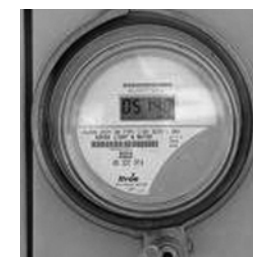
We'll soon be installing digital (electronic) meters like these.
